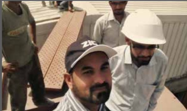
Deep penetrating test of bottom plate tanks being done under the supervision of HTBL employees
