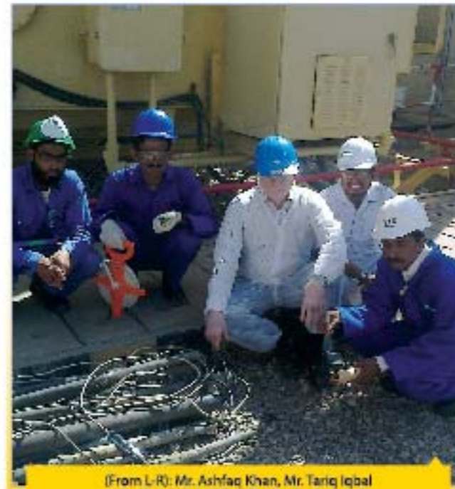
(From L-R): Mr. Ashfaq Khan, Mr. Tariq Iqbal, Mr. Abdul Wahid Suddle, Mr. Rashid and Mr. Aqeel Ahmed at HUBCO Power Plant
