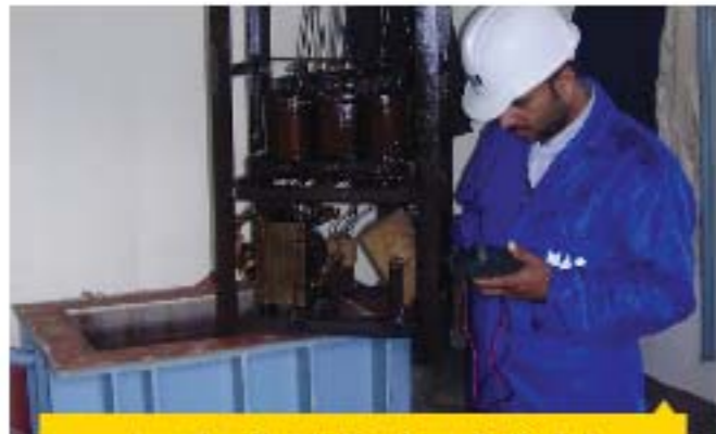
Inspection of Installed Transformer Rectifier Unit
